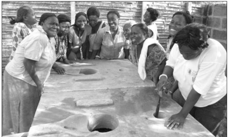
Women are finishing up the cement base they made for the composting toilet.
